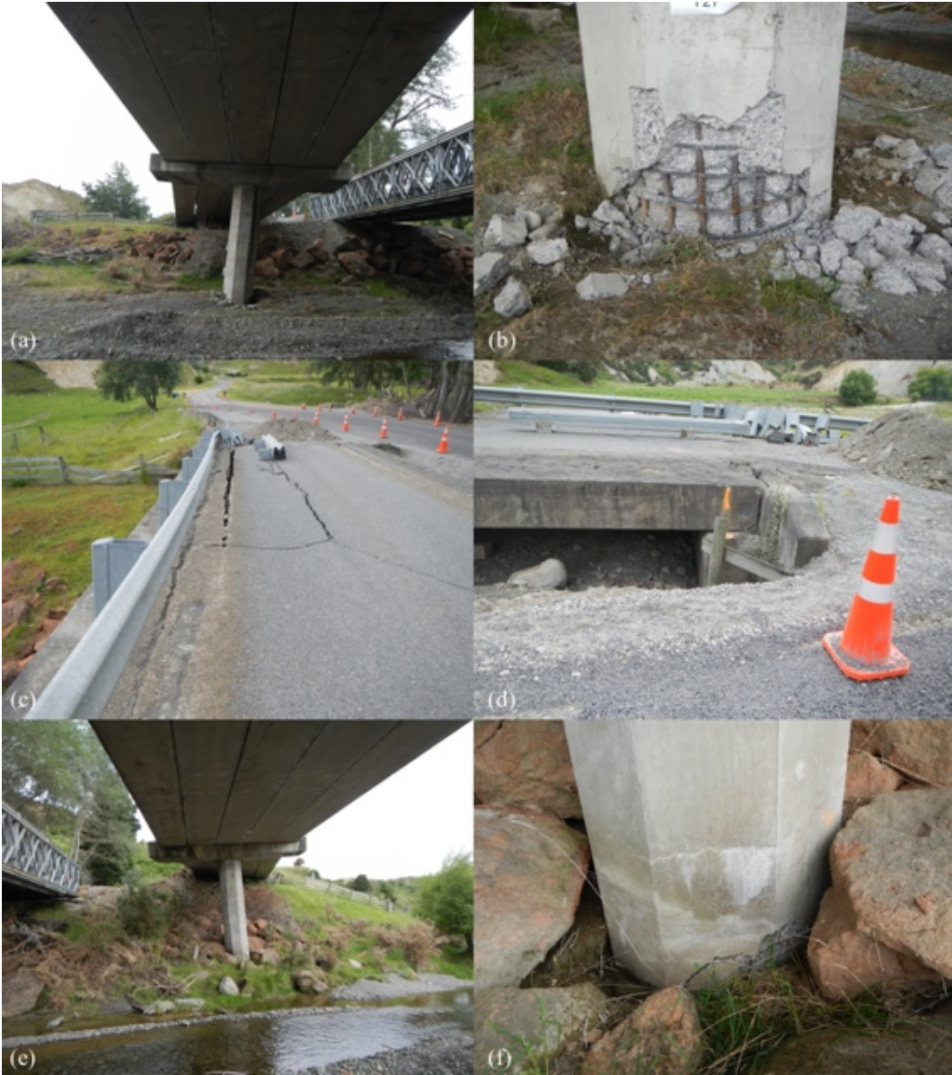
Figure 6.30: Structural damage to Wandle Bridge [-42.5864, 173.1003]: (a) South approach from under bridge; (b) Plastic hinging on pier near south approach; (c) Deck at southern end; (d) South abutment; (e) North approach from under bridge; (f) Minor hinging on pier near north abutment.
