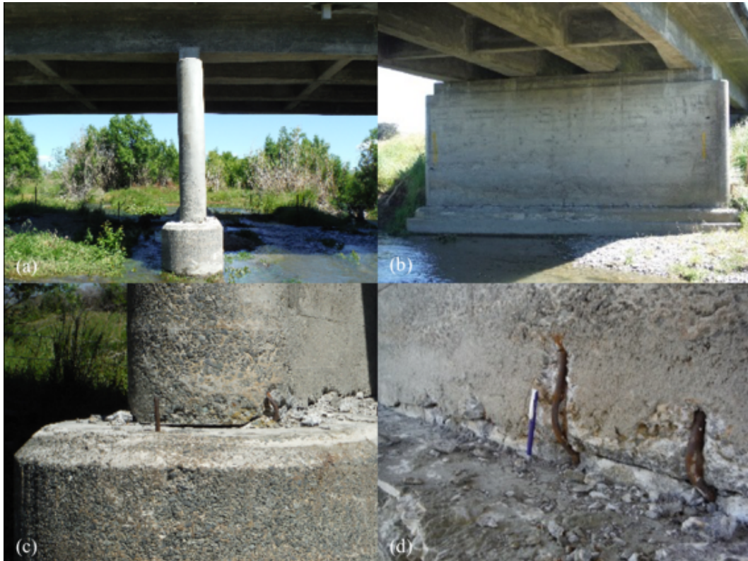
Figure 6.48: Substructure damage at Flaxbourne River Bridge [-41.8085, 174.1458]: (a) Tilted pier; (b) Cracking at pier base; (c) and (d) Cracking and exposed reinforcement at base of piers.
