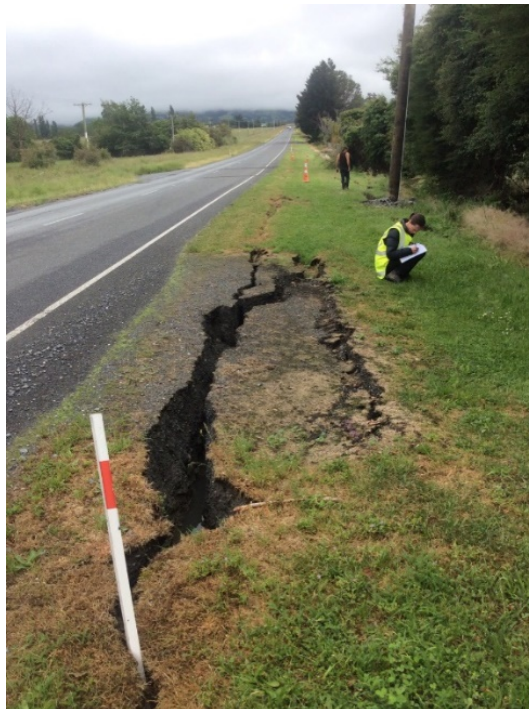
Figure 6.77: Lateral spreading cracks at the side of Athelney Road (9 Dec 2016, facing north) [-42.3598, 173.6765]. Note the drainage ditch to the right of the photo.
