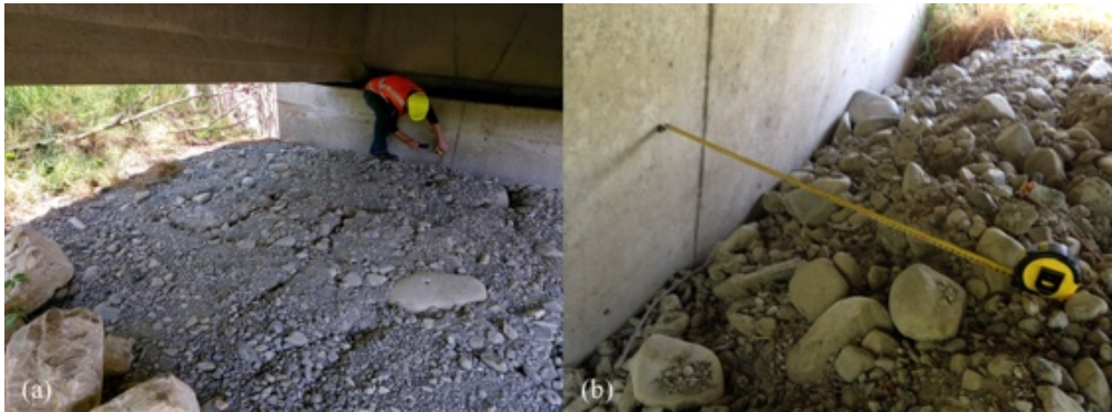
Figure 6.23: Cracking and gapping in fill below bridge deck at northern abutment to Lower Mason Bridge indicating riverward movement of the fill [-42.6334, 173.0666]: (a) Looking north; (b) 60 cm gap between wall and fill.
