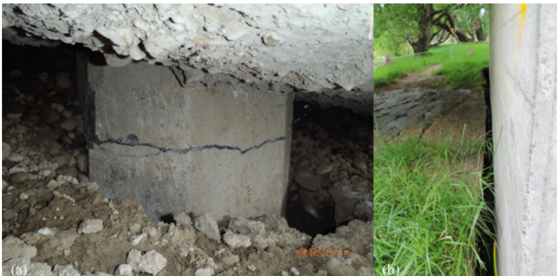
Figure 6.54: Pile and footing damage at Needles Creek Bridge [-41.8217, 174.1370]: (a) Crack in pile for south abutment; (b) Soil-footing gapping at pier 3.
