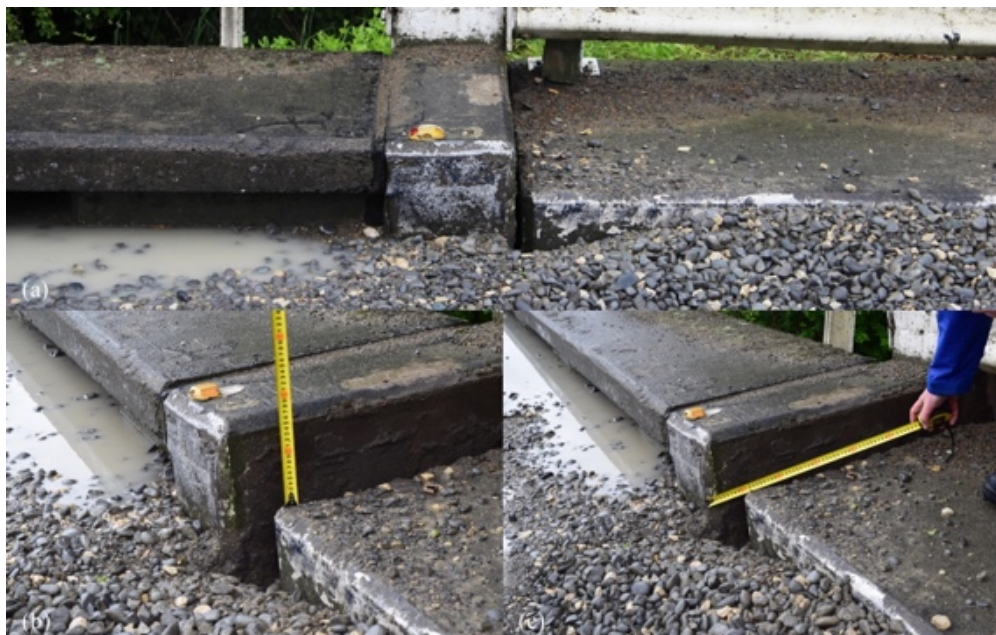
Figure 6.13: Settlement and outward movement at north side of eastern abutment to Waiiau River Bridge as indicated by offset of concrete members [-42.6552, 173.037].
