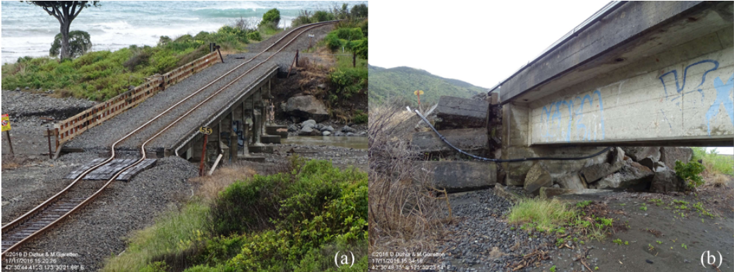
Figure 6.86: Damage at Oaro River Rail Bridge [-42.514025, 173.50682]: (a) Residual lateral deformation towards the east at the northern abutment has bent the tracks (photo looking south); (b) Northern abutment looking north. Photos courtesy of D. Dizhur and M. Giaretton.
