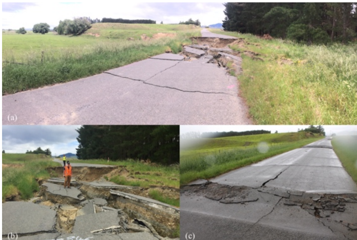
Figure 6.39: Failure and severe cracking on Leslie Hills Road (photos all taken looking west) [-42.6306,172.9895]: (a) Overview of major failure area; (b) Closer view of failure area; (c) Cracking to west of failure area.
