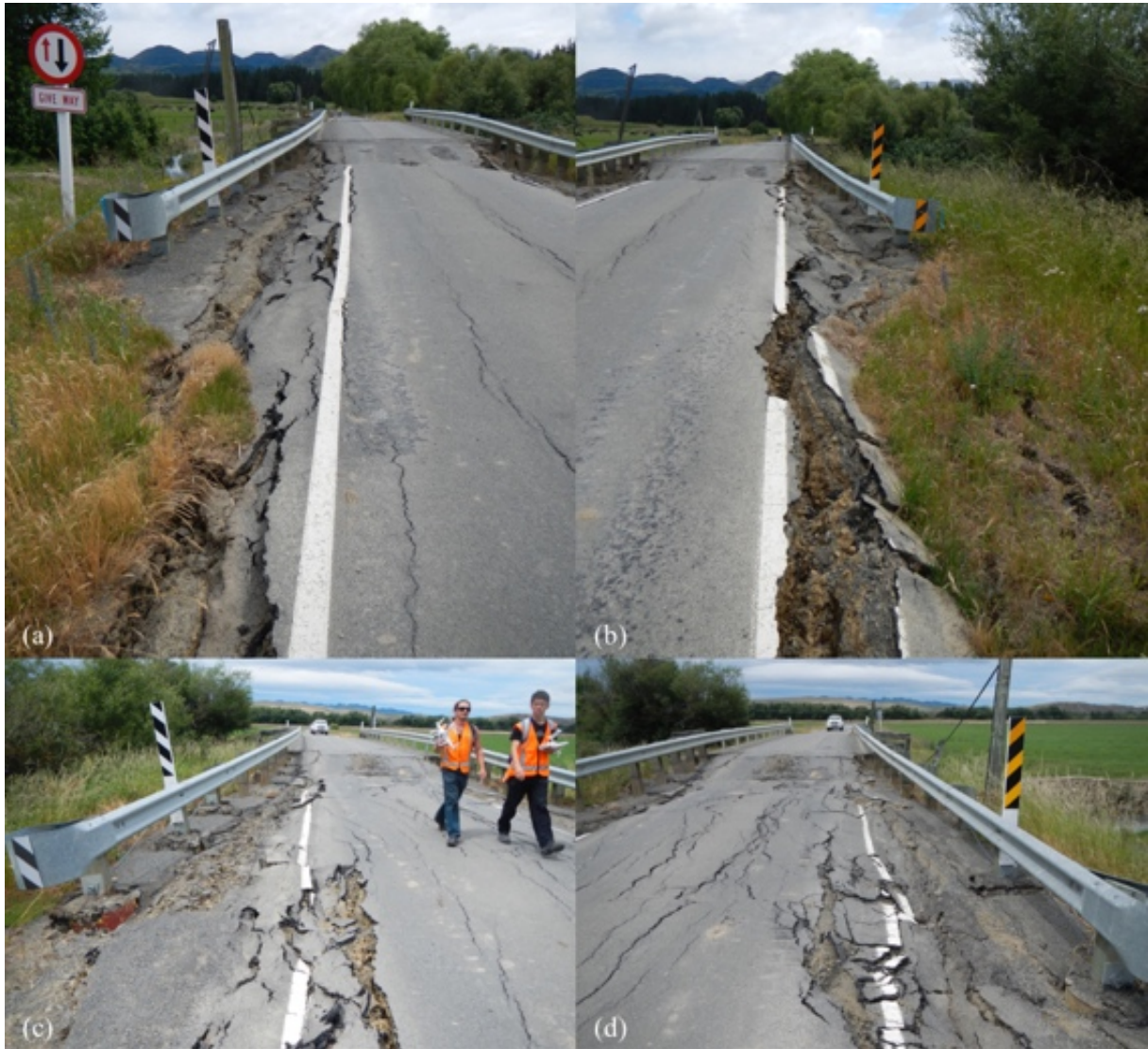
Figure 6.44: Settlement and cracking in approaches to Mt Paul Bridge [-42.6355, 172.9924]: (a) Southwest corner; (b) Southeast corner; (c) Northeast corner; (d) Northwest corner.
