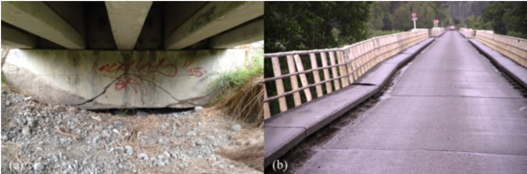
Figure 6.7: Structural damage at western approach area to Waiau River Bridge [-42.6556, 173.0302]: (a) Severe cracking in the abutment wall (looking west from under the bridge deck); (b) Differential settlement at second pier (looking east).
