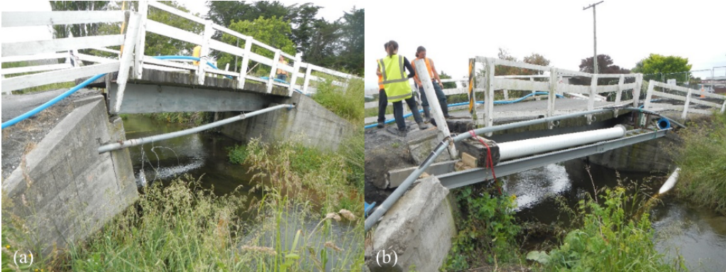
Figure 6.66: Back rotation of east and west abutments at Lyell Creek Bridge [-42.3892, 173.6773]: (a) Looking south at bridge; (b) Looking north at bridge.
