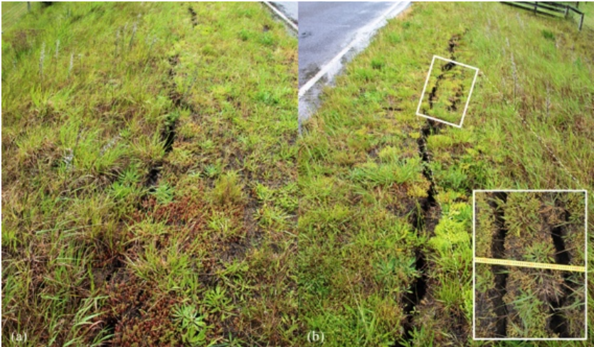
Figure 6.15: Cracks along edges of the western approach embankment for Mason Bridge (looking east towards bridge) [-42.6464, 173.04196]: (a) North side; (b) South side – inset shows close-up of cracks as indicated.
