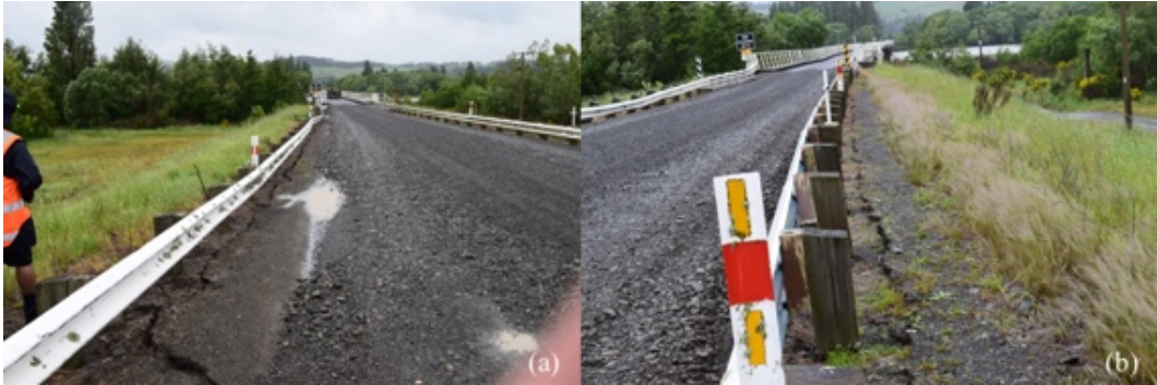
Figure 6.3: Lateral cracking on road side in western approach embankment of Waiiau River Bridge. Photos taken looking east towards bridge [-42.6556, 173.0294]: (a) North side; (b) South side.
