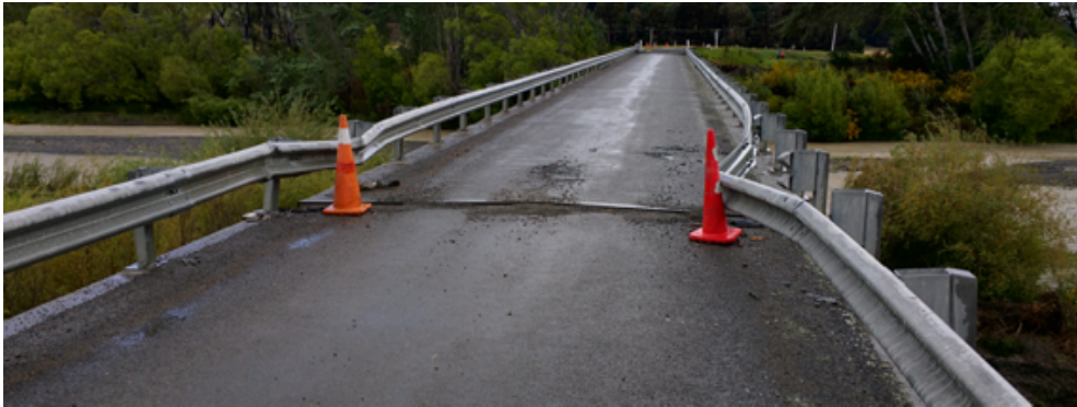
Figure 6.25: Buckling of guard rails at centre expansion joint of Lower Mason Bridge indicating that the two main deck sections have undergone permanent inward deformation. Photo facing south [-42.6343, 173.0664].
