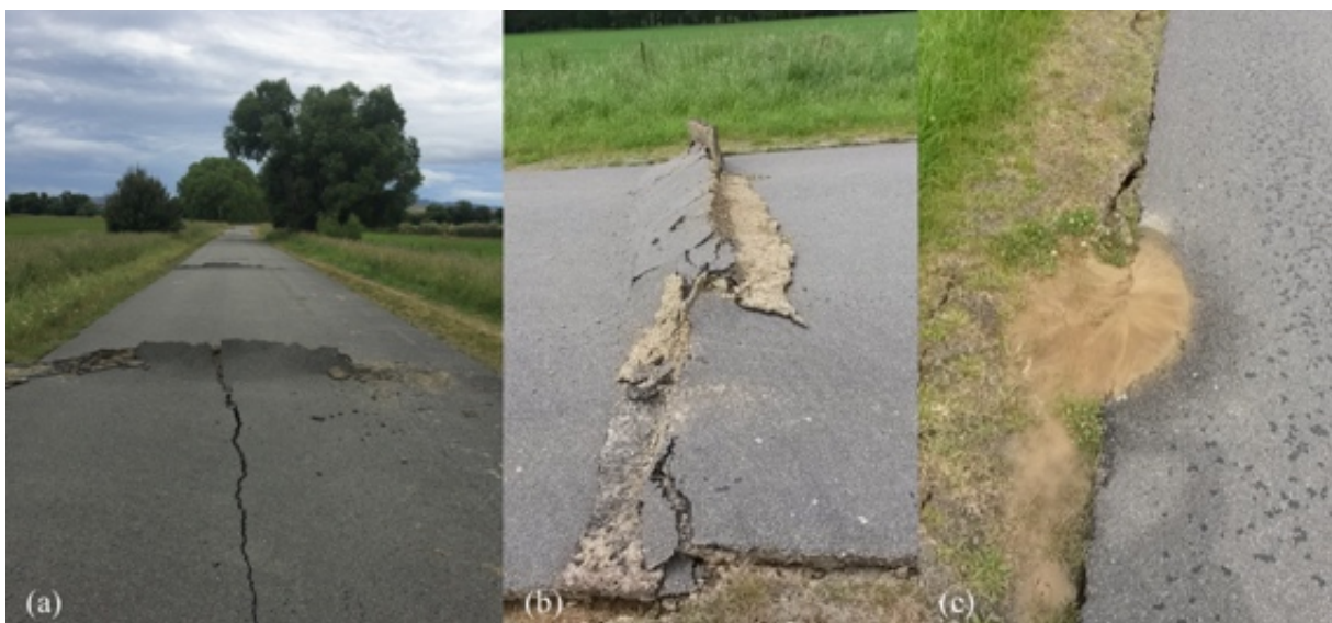
Figure 6.41: Damage observations east of Leslie Hills Road failure area [-42.6306,172.9895]: (a) Compression ridging in pavement material; (b) Side view of compression ridge; (c) Minor liquefaction ejecta.
