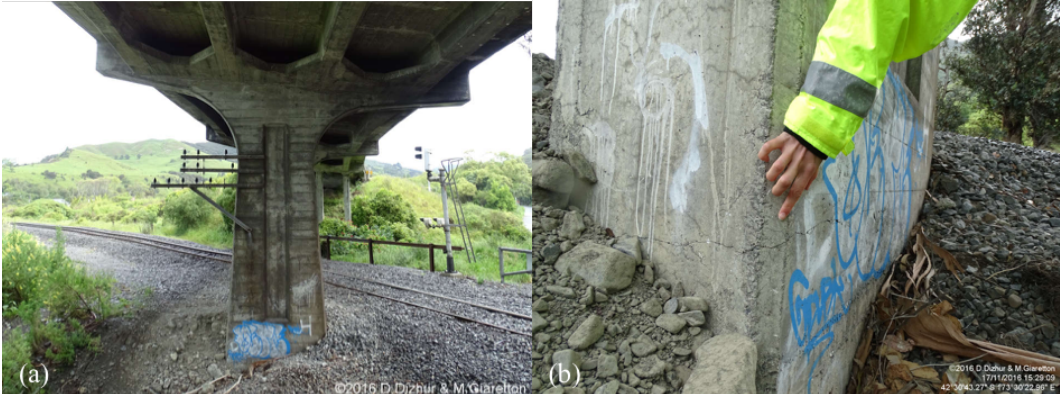
Figure 6.85: Damage at Oaro Overbridge [-42.512089, 173.506345]: (a) Northernmost central hammerhead pier looking south; (b) Flexural cracking at base of northernmost hammerhead pier. Photos courtesy of D. Dizhur and M. Giaretton.
