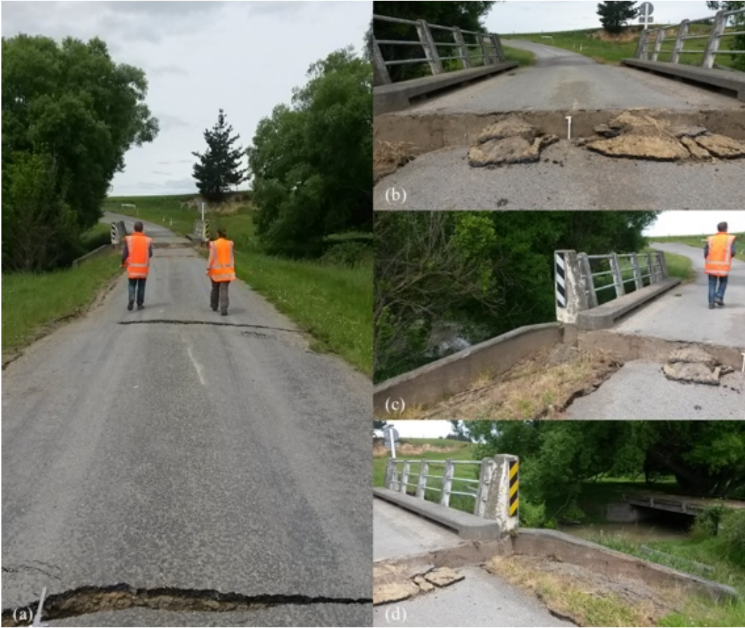
Figure 6.38: Home Creek Bridge [-42.6323, 172.9528]: (a) Roadway cracks in western approach; (b), (c), and (d) Settlement at western abutment.
