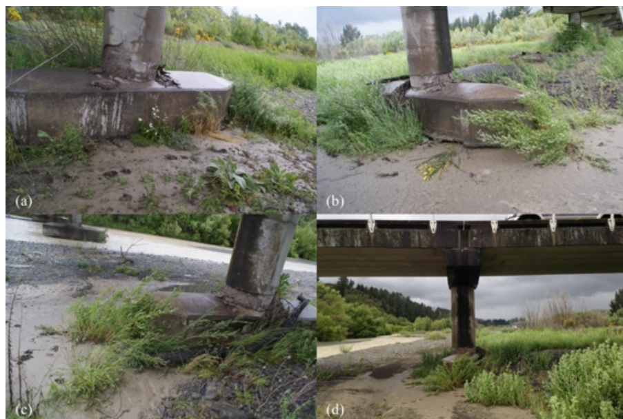
Figure 6.18: Ejecta near bridge piers and footings at Mason Bridge [-42.647, 173.043]: (a) Looking east; (b) Looking north; (c) Looking west; (d) Looking north.
