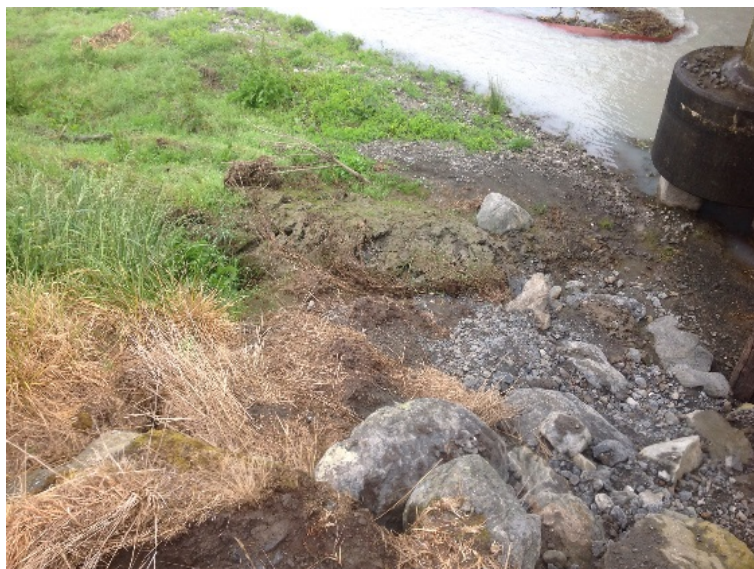
Figure 6.70: Liquefaction close to the north pier and abutment of Middle Creek Railway Bridge (facing southeast) [-42.3670, 173.6861].
