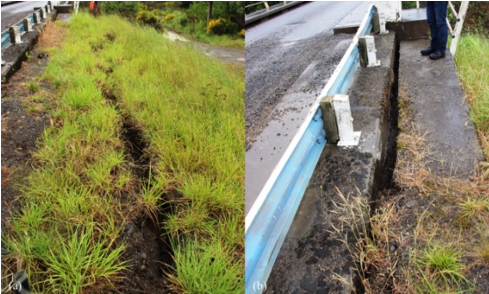
Figure 6.4: South side of western approach embankment to Waiiau River Bridge [-42.6556, 173.03]: (a) Lateral cracks in embankment side; (b) Settlement and outward movement at abutment wall.
