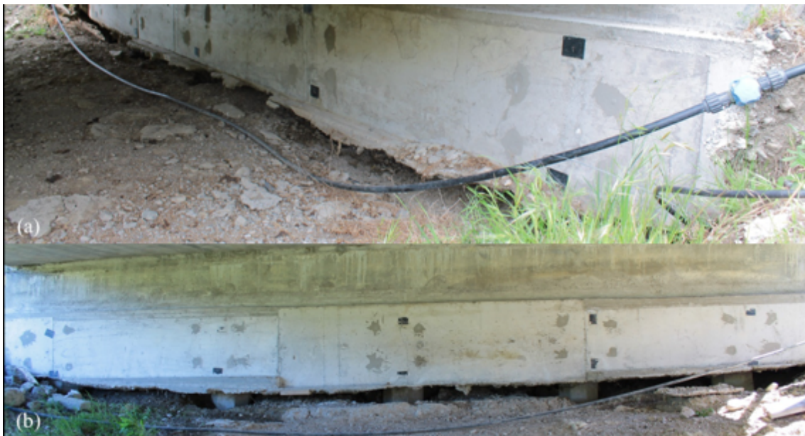
Figure 6.53: Soil subsidence below abutments at Needles Creek Bridge [-41.8217, 174.1370]: (a) North abutment wall looking northwest; (b) South abutment wall looking south.
