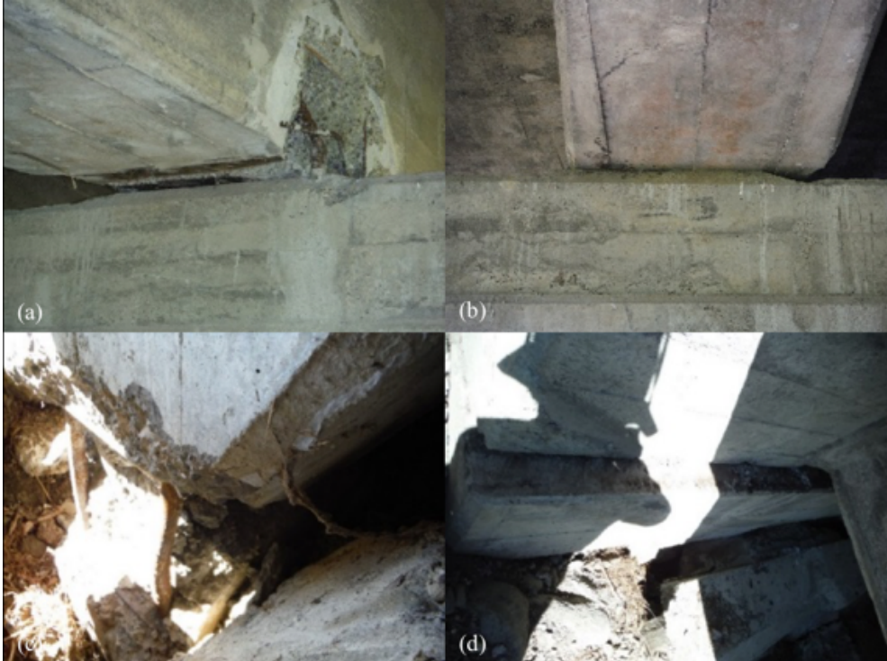
Figure 6.47: Damage at Flaxbourne River Bridge [-41.8085, 174.1458]: (a) Damage at deck-pier connection; (b) Residual transverse deck displacement; (c) Exposed and buckled reinforcement in abutment columns; (d) Residual longitudinal deck displacement.
