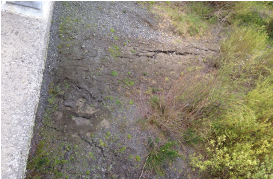
Figure 6.26: Cracks in northern river bank on eastern side of bridge. Photo taken from bridge deck. Riverward direction is down for this orientation [-42.6342, 173.0665].
