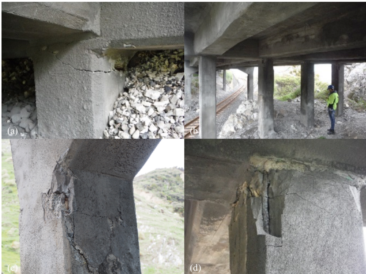
Figure 6.61: Structural damage observations at the Mororimu Overbridge [-42.2166, 173.8686]: (a) Abutment column cracking; (b) Damage to pier columns; (c) Cracking below knee joint of central pier column; (d) Exposed reinforcement at top of pier column.
