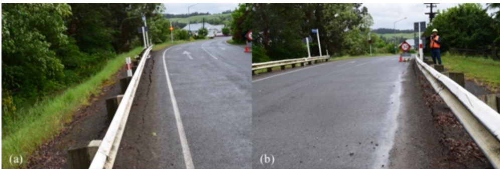
Figure 6.12: Lateral cracking on both sides of roadway in eastern approach embankment to Waiiau River Bridge [-42.6551, 173.0380]: (a) Northern side (looking east away from bridge); (b) Southern side (looking east).
