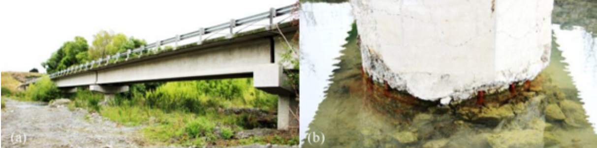
Figure 6.31: Lottery River Bridge [-42.6097, 173.0854]: (a) General layout; (b) Plastic hinge damage at base of pier.
