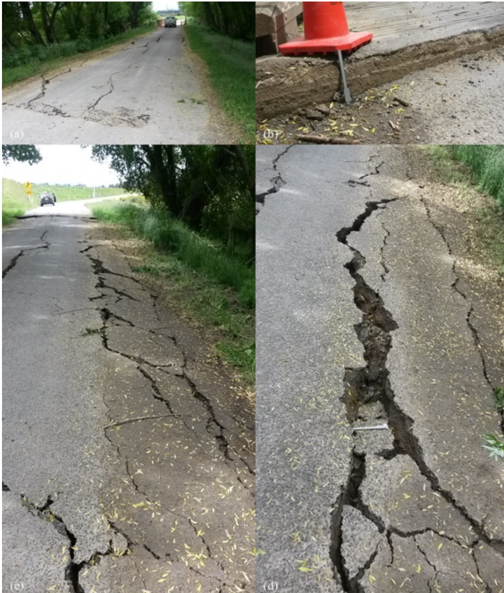
Figure 6.45: Damage at Emu Plains Bridge [-42.6394, 172.9149]: (a) Roadway damage looking west towards bridge; (b) Settlement at eastern abutment; (c) and (d) Significant cracking in roadway on eastern side of bridge (photos taken facing east away from bridge).
