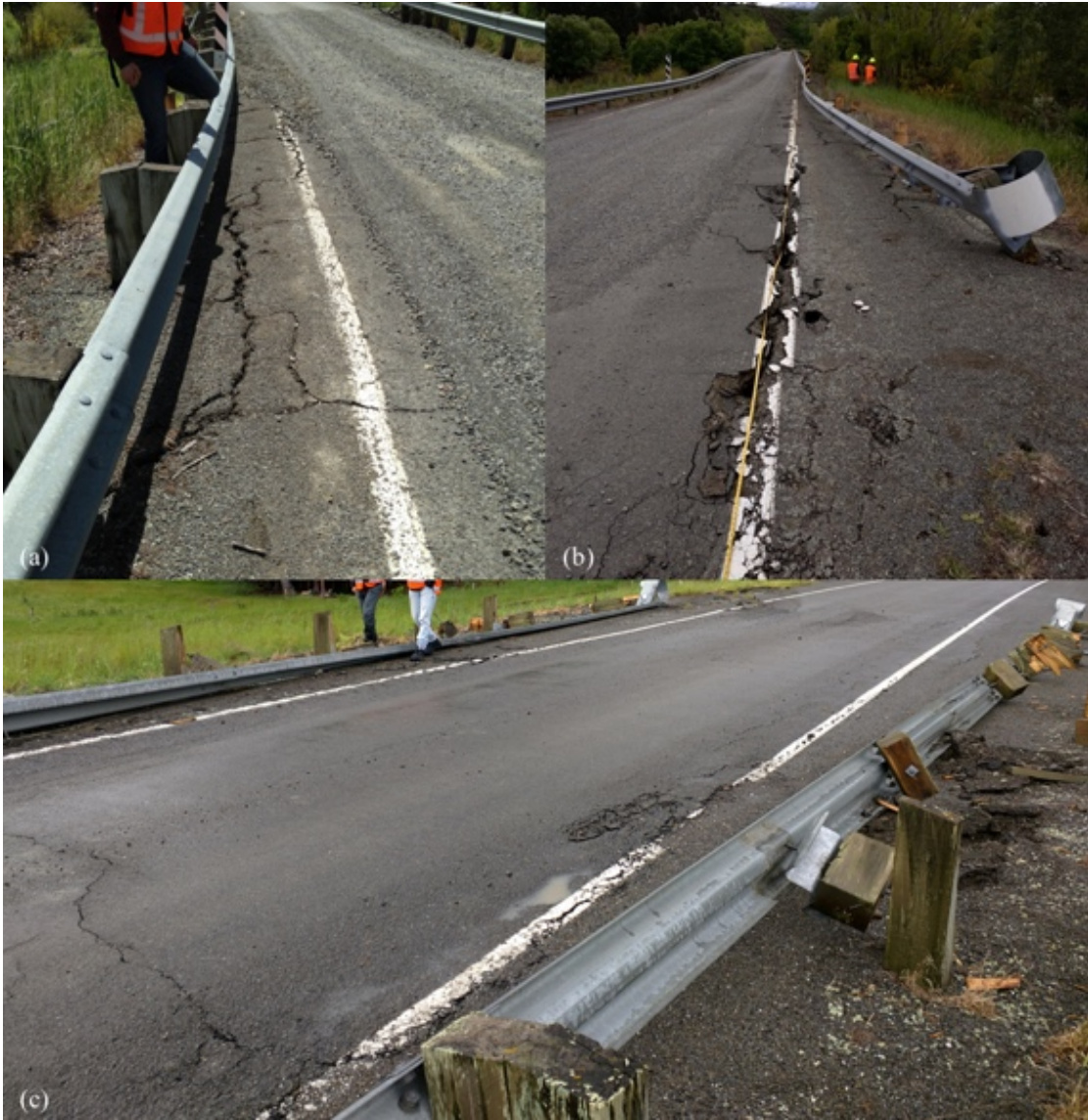
Figure 6.20: Cracking in approach roadways at Lower Mason Bridge: (a) Western side of south approach looking north [-42.6353, 173.0662]; (b) Eastern side of south approach looking north [-42.6353, 173.0662]; (c) North approach looking northwest across road [-42.6330, 173.0666].
