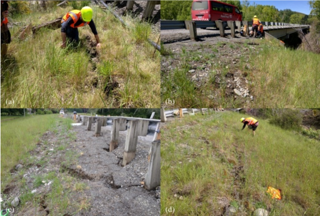
Figure 6.21: Cracking in sides of approach embankments at Lower Mason Bridge. (a) West side of south approach looking north [-42.6353, 173.0662]; (b) East side of south approach looking north [-42.6353, 173.0662]; (c) and (d) West side of north approach looking north and south, respectively [-42.6330, 173.0666].
