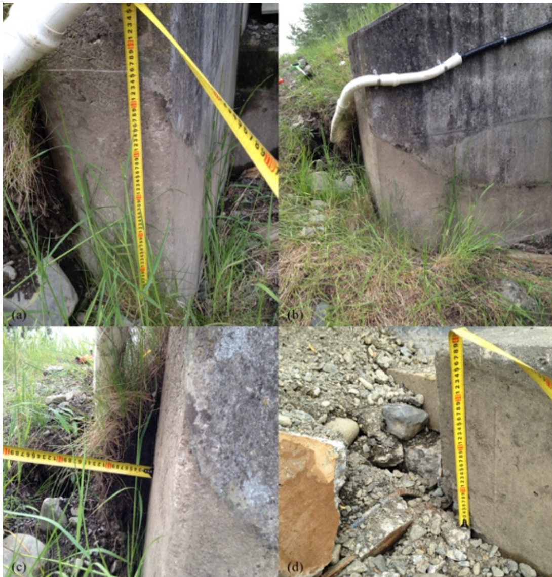
Figure 6.22: Settlement and outward movement at west side of north abutment to Lower Mason Bridge [-42.6334, 173.0666]: (a) Edge of abutment wall looking east; (b) Abutment wall looking north; (c) Edge of abutment wall looking north; (d) Embankment side of abutment wall near deck connection looking south.
