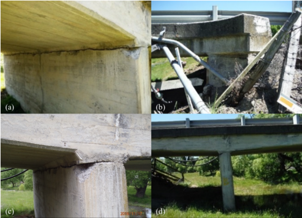
Figure 6.55: Structural damage at Needles Creek Bridge [-41.8217, 174.1370]: (a) Cracking across length of pier 1 looking south; (b) Deck sheared off of abutment 1 facing west; (c) Cracking at pier 1 facing east; (d) Tilting of pier 1 facing east.
