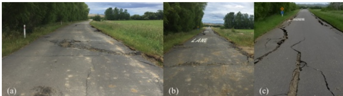
Figure 6.42: Cracking in roadway approaching Mt Paul Bridge from the north along Leslie Hills Road [-42.6355, 172.9924].
