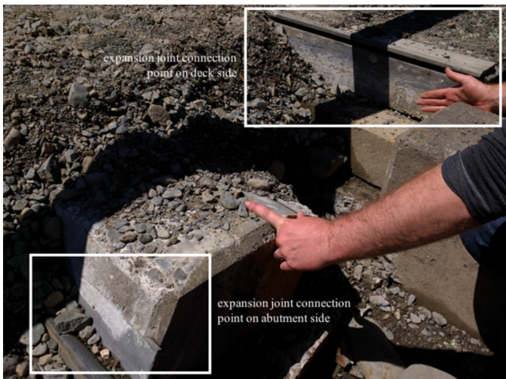
Figure 6.24: Damage to abutment-deck connection at Lower Mason Bridge due to relative movement of abutment wall and deck. The breakaway member to the left was pushed back away from the deck and rotated 180° such that the connection point for the expansion joint faces away from the deck [-42.6334, 173.0666].
