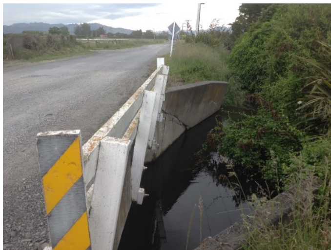
Figure 6.82: Failure of the northwest wingwall of the Lyell Creek culvert on Mill Road (8 Dec 2016, facing west) [-42.3765, 173.6788].
