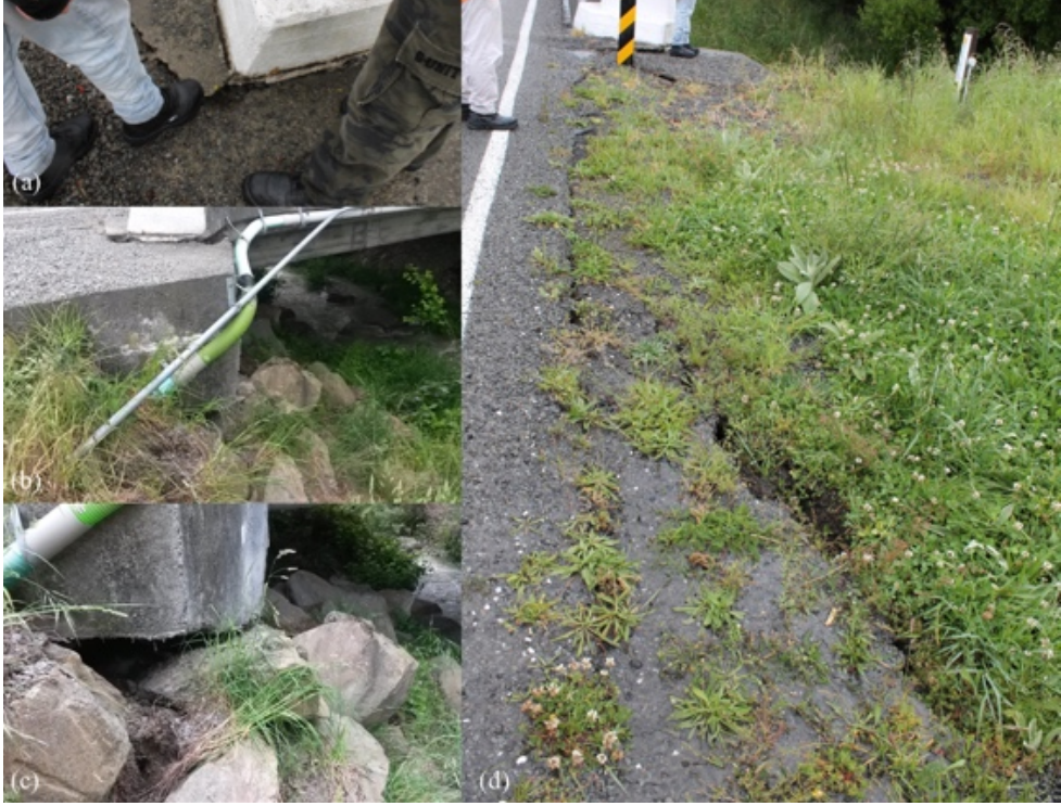
Figure 6.36: West corner of Stinking Stream Bridge [-42.672427, 172.774764]: (a) Settlement and cracking at abutment; (b) Settlement looking east; (c) Rip-rap movement away from the abutment base; (d) Cracking in approach.
