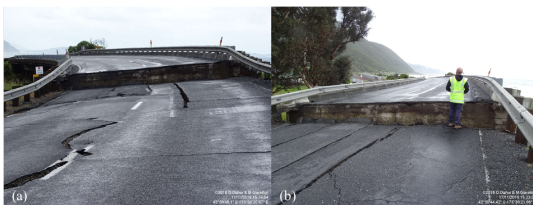
Figure 6.83: Settlement and severe approach roadway cracking at southern abutment to Oaro Overbridge [-42.5121, 173.5063] looking north. Photos by D. Dizhur and M. Giaretton.
