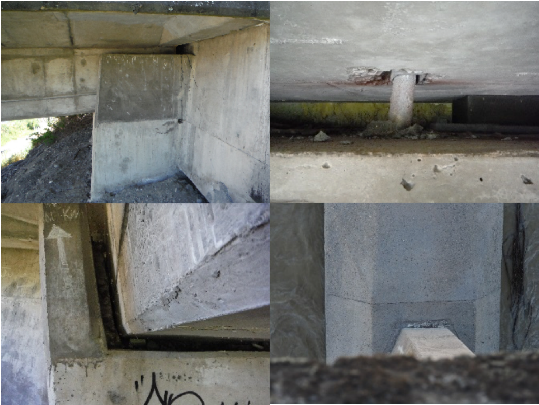
Figure 6.62: Structural damage at Clarence River Bridge [-42.1592, 173.9103]: (a) Cracking in transverse abutment wall; (b) Residual deformation in hold down rod securing deck to abutment; (c) Deck settlement at abutment; (d) Concrete spalling at base of pier.
