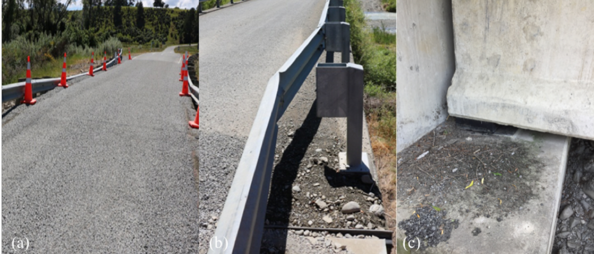
Figure 6.32: Damage at Lottery River Bridge [-42.6097, 173.0854]: (a) Gravel in-fill due to settlement and guardrail damage at northeast approach looking northeast; (b) Residual transverse offset of deck and abutment at northeast abutment looking southwest; (c) Residual displacement of bearing pad at southwest abutment looking west.
