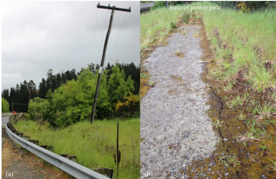
Figure 6.16: Northern side of eastern approach to Mason Bridge (looking west) [-42.6475, 173.04465]: (a) Power pole has moved down the slope of an embankment directly adjacent to bridge approach embankment; (b) Cracks parallel to roadway in embankment fill.
