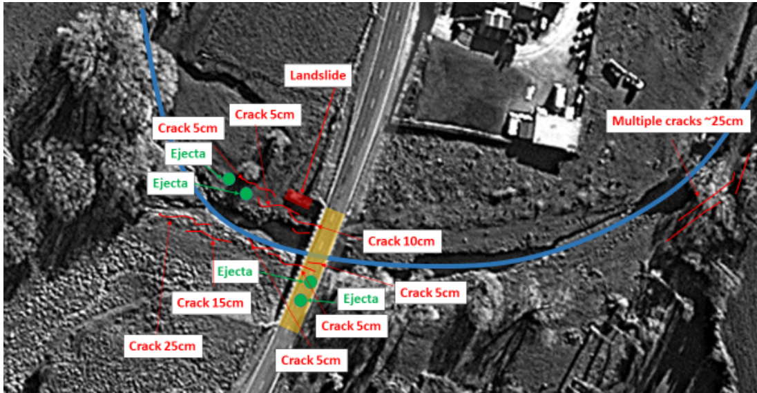
Figure 6.50: Overview of Needles Creek Bridge site with indications of ground damage. Orange area is the bridge deck, red lines indicate cracks, and the green markers indicate sand boils. The blue line indicates the creek bed.
