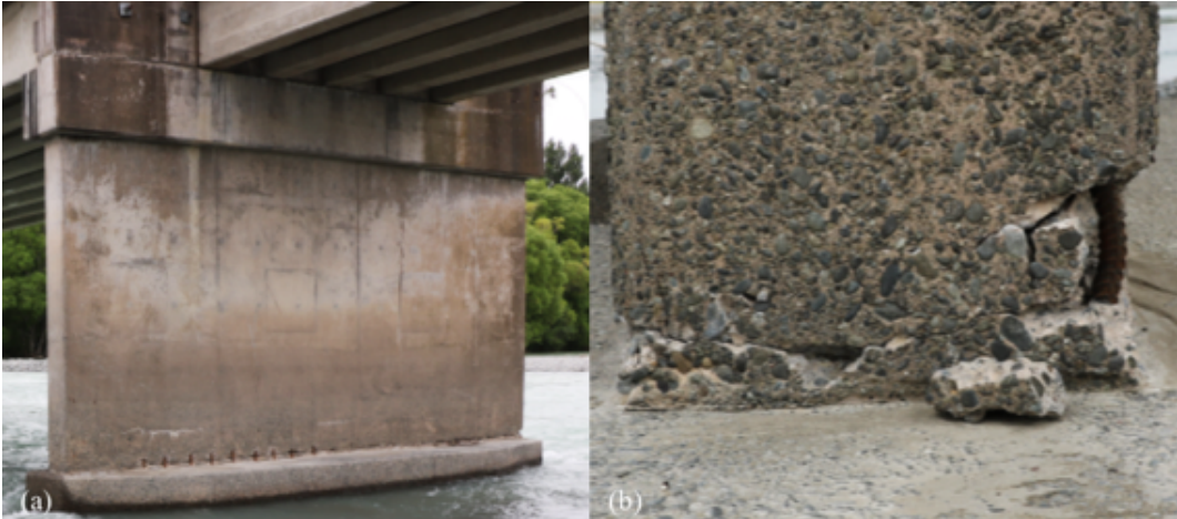
Figure 6.8: Structural damage to base of piers for Waiau River Bridge [-42.6553, 173.0351]: (a) Cracking at pile cap interface; (b) Exposure and buckling of longitudinal bars.
