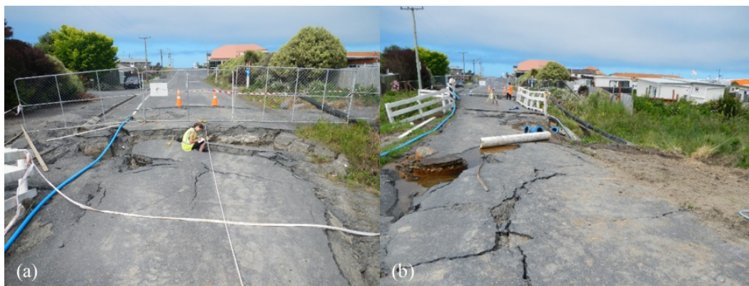
Figure 6.65: Approach cracking at Lyell Creek Bridge [-42.3892, 173.6773]: (a) Eastern approach looking east; Note: crack at 9, from the bridge abutment (location of field member) was 50 cm wide, and had a vertical offset of 30 cm. (b) Western approach looking east.
