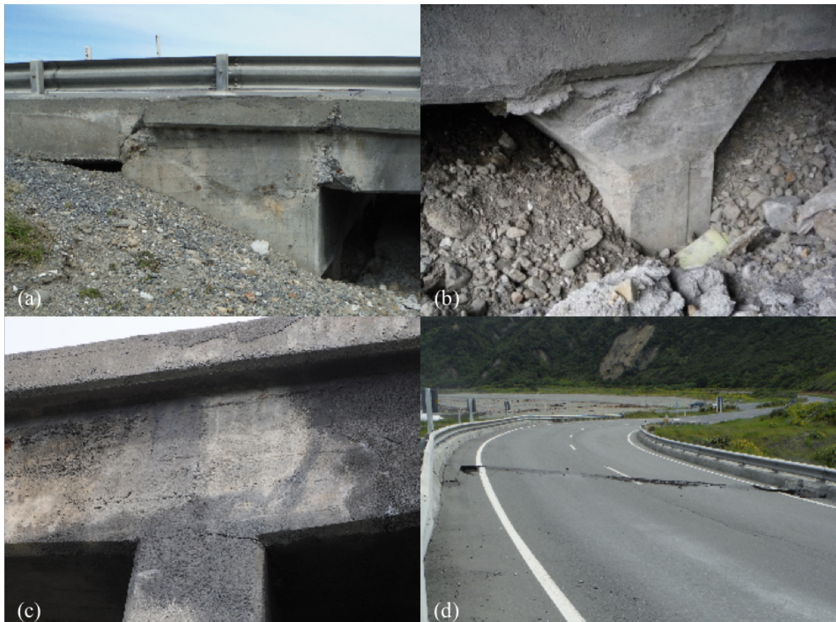
Figure 6.60: Damage observed at Mororimu Stream Bridge [-42.2173, 173.8673]: (a) Cracking in eastern abutment looking south; (b) Abutment column cracking; (c) Cracking at top of pier; (d) Settlement of eastern approach looking west.
