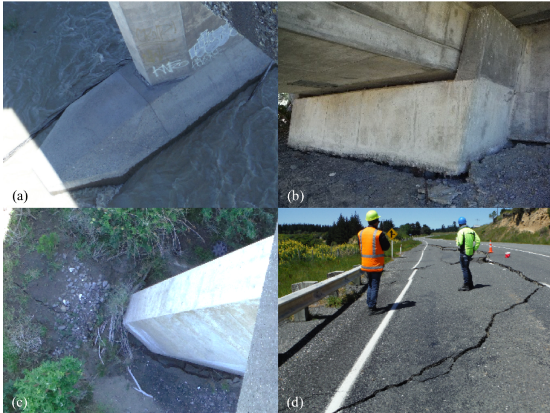
Figure 6.63: Damage at Clarence River Bridge [-42.1592, 173.9103]: (a) Cracking in top of footing; (b) Settlement of fill ahead of abutment; (c) Soil gapping at base of pier; (d) Spreading cracks in roadway at southern approach looking south.
