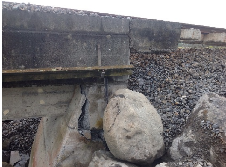
Figure 6.72: Damage to the north abutment of the Middle Creek Railway Bridge facing northwest [-42.3670, 173.6861].
