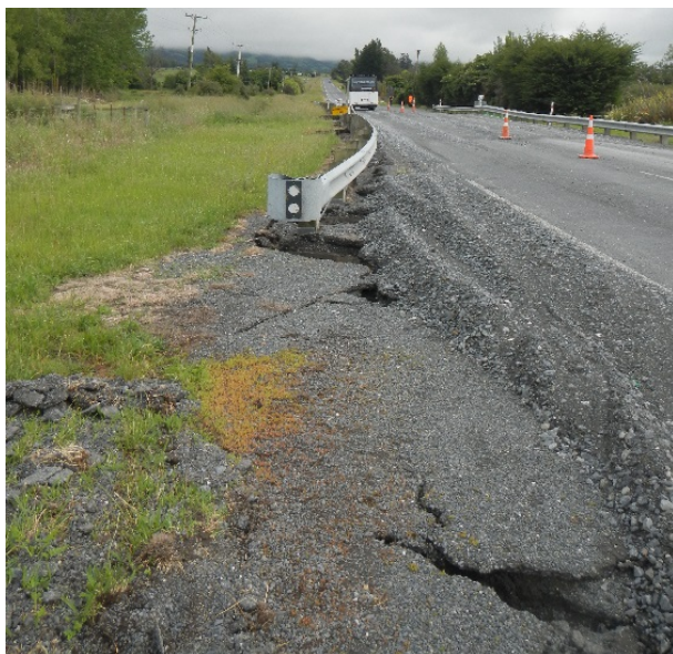
Figure 6.79: Cracking on the south side of the Waimagarara culvert on Athelney Road (9 Dec 2016, facing north) [-42.3606, 173.6765].
