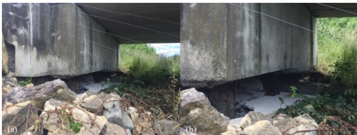
Figure 6.43: Settlement below abutment at Mt Paul Bridge [-42.6355, 172.9923].
