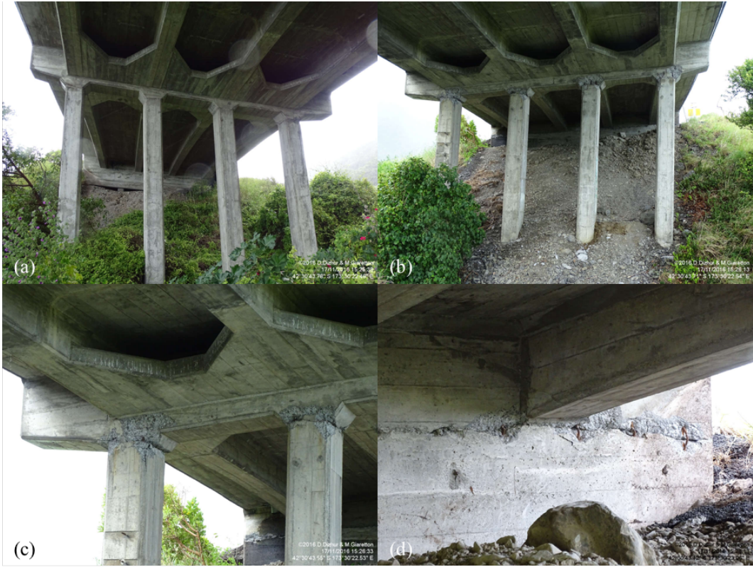
Figure 6.84: Damage at Oaro Overbridge [-42.5121, 173.5063]: (a) Settlement of fill ahead of southern abutment and cracking at top of pier columns looking south; (b) Cracking in fill ahead of northern abutment and plastic hinging at top of pier columns looking north; (c) Closer view of damage at top of pier columns in northernmost pier looking north; (d) Cracking across face of northern abutment wall, just below deck beams looking north. Photos courtesy of D. Dizhur and M. Giaretton.
