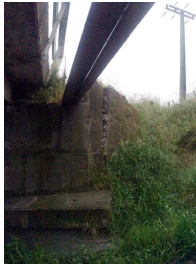
Figure 6.75: Damage to the north abutment on the east side of the bridge (8 Dec 2016, facing north) [-42.3692, 173.6549].
