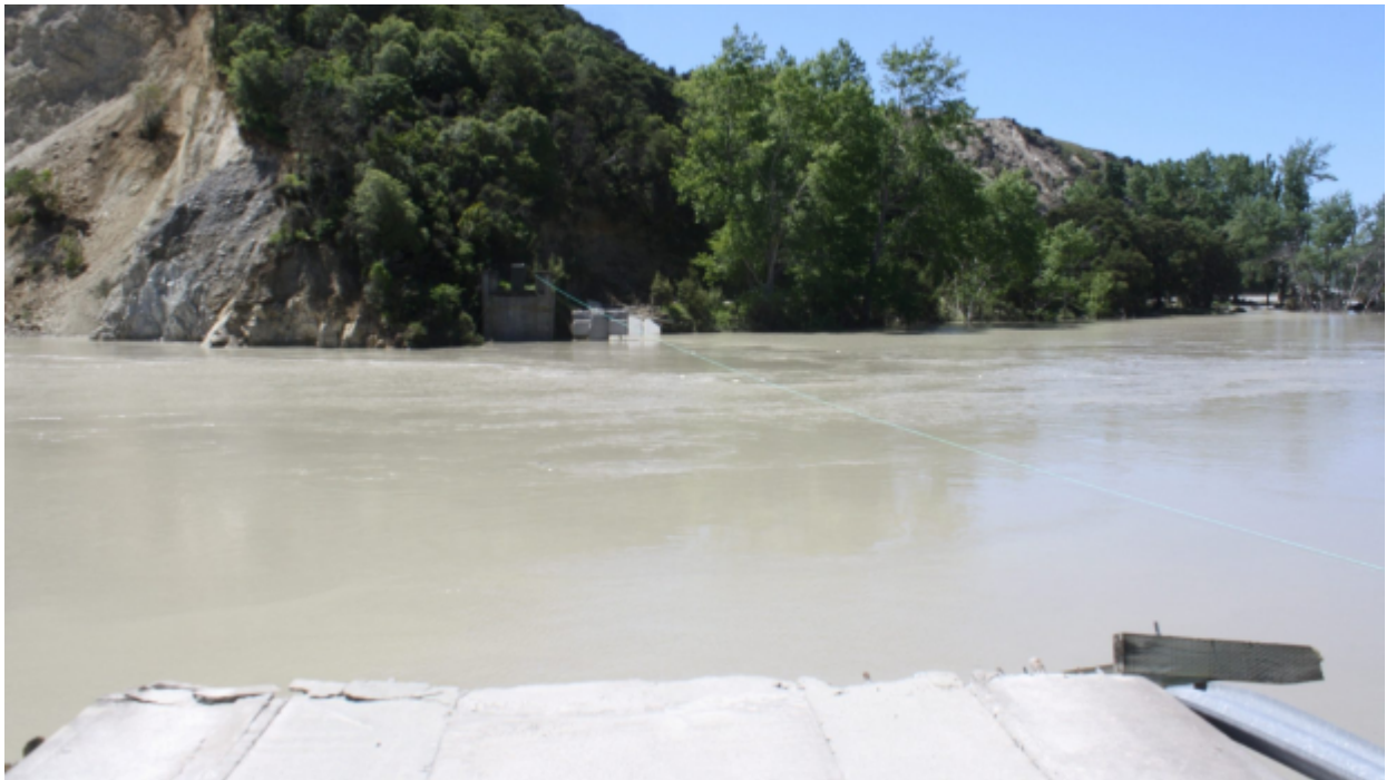
Figure 6.87: Collapse of Clarence Valley Road Bridge [-42.11066, 173.84156]. Photo taken from western side looking east (stuff.co.nz, 2016).
